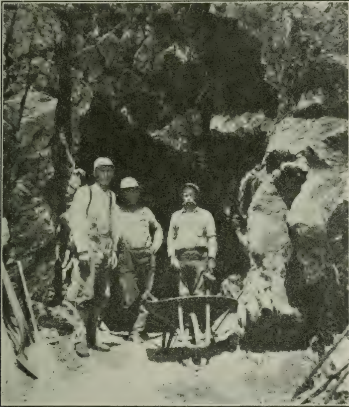
Photo No. 34. Tunnel at Noble Electric Steel Company's Red Mountain lease, driven to crosscut ledge shown in Photo No. 33.
